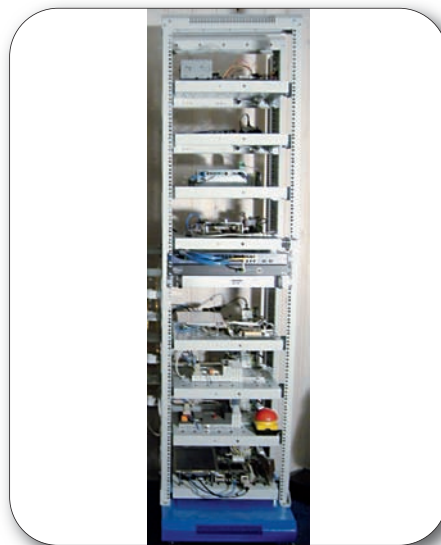
Figure 1. Each test rack in the OSADL QA farm has eight power switches with a network connection, eight network switches (10/100/1000 Mbit/s) with port mirroring, and eight serial network adapters.
